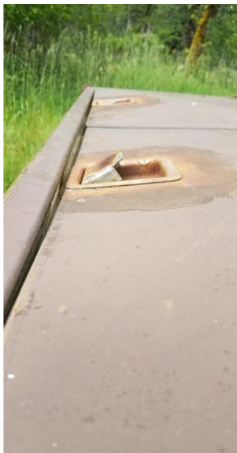
Photo 8: Johnson Bar Campground—this dumpster lever is rusted in the open position
